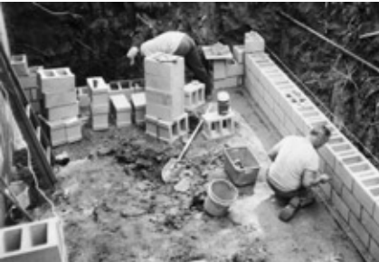
Peter Bergs (back) and Jim Voight work on the new foundation for the Red Wing addition
